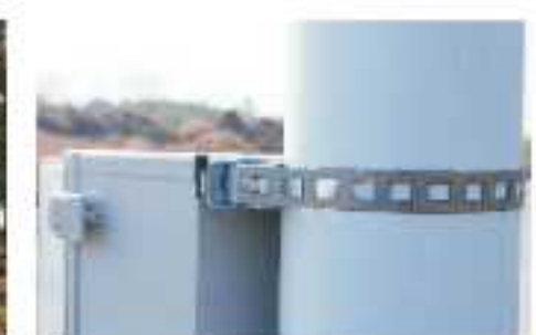
Fixed on the telegraph pole
