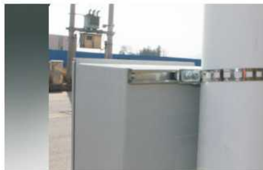
Fixed on the telegraph pole
