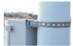
Fixed on the telegraph pole
